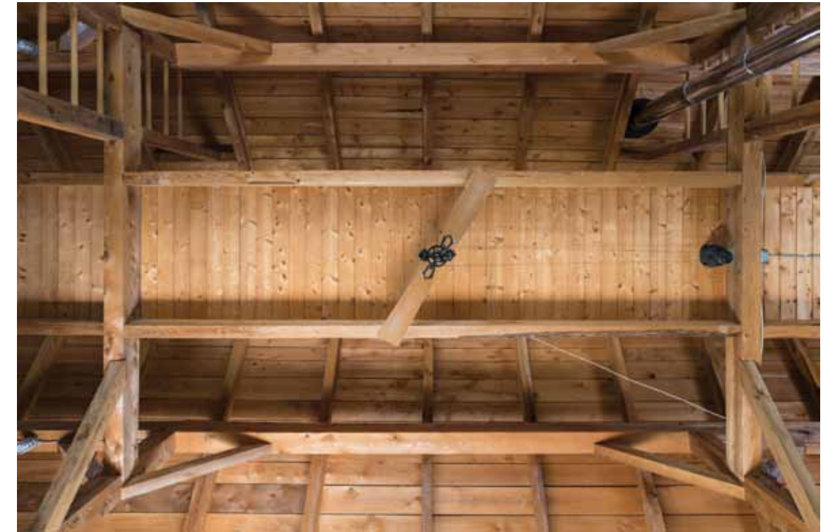
A view of the interior of the post-and-beam home (opposite) with hemlock framing, kitchen, and master bedroom in the upstairs hayloft. The ladder to the left is made of hemlock and ash. The gray barn-board walls are from Carlisle Wide Plank Floors. The new kitchen hutch was built to look like a family heirloom.
